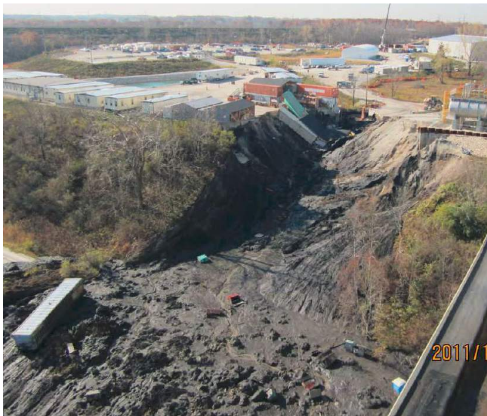
October, 2011 bluff failure at We Energies Oak Creek Power Plant. Source: WDNR & We Energies
